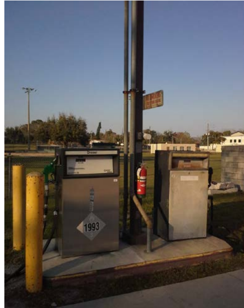
Fuel Pumps Installed in 1991 (28 years ago)
